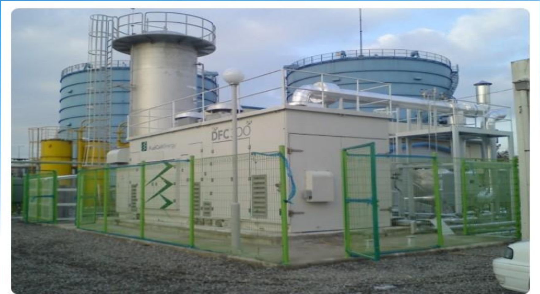
Electrical & Instrument Work for Fuel cell Pilot of SK Gas Co. Korea / Completion 2018
