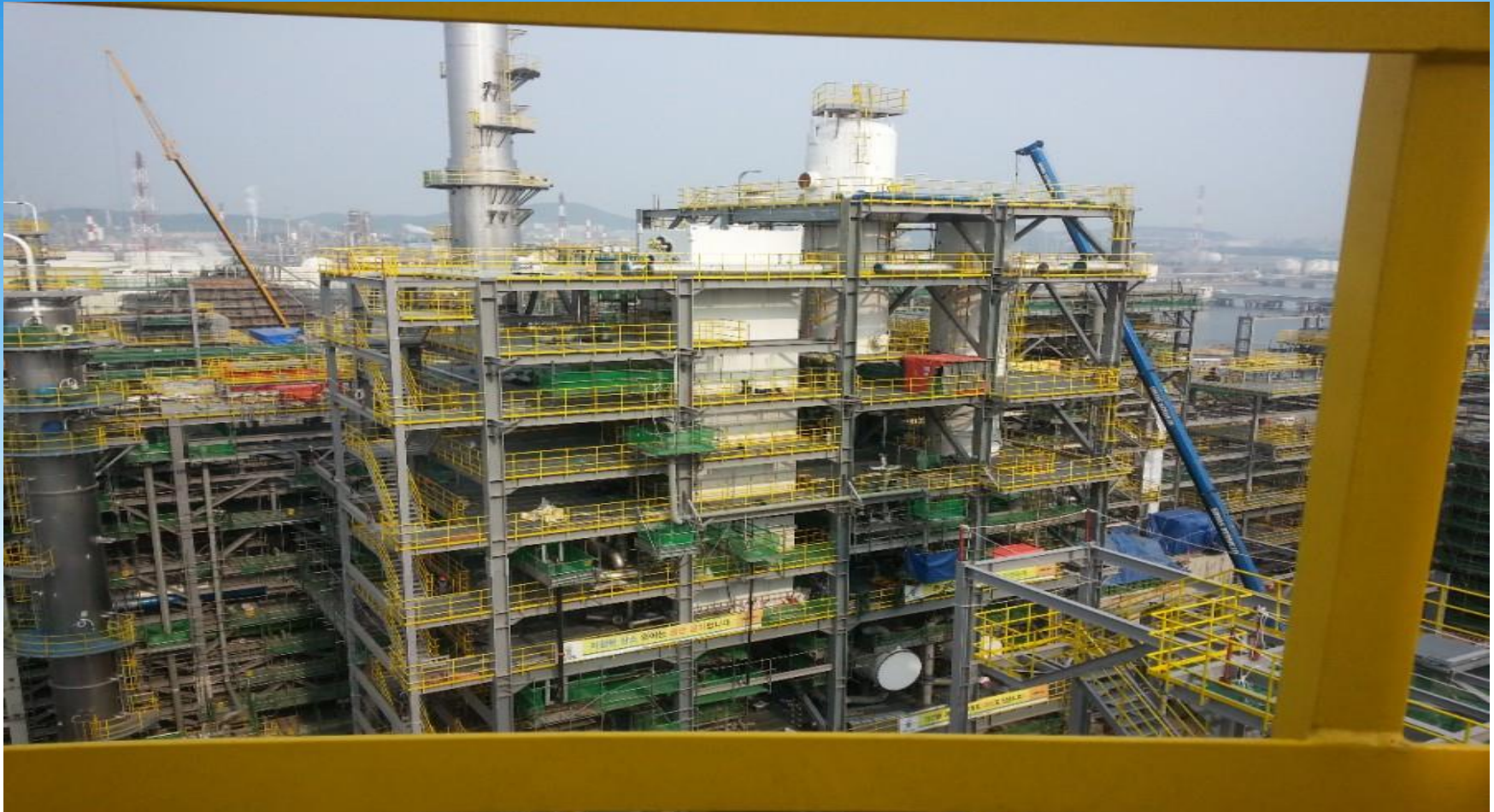
Electrical & Instrument Work for S-oil Super Project Package #3, Korea / Completion 2017
