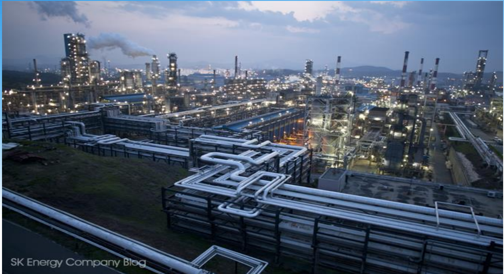
Electrical & Instrument Work for New PX Project (OBL) in SK Energy Ulsan Site, Korea / Completion 2014
